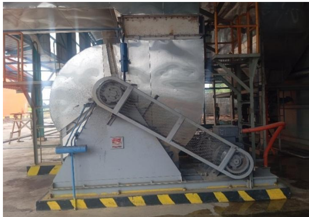
Gambar 6 Blower Induced Draft Fan
